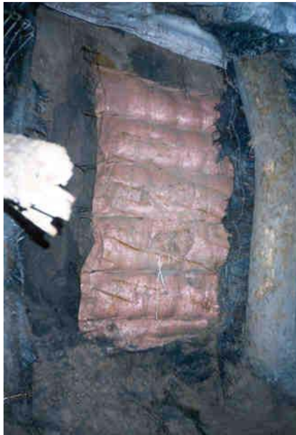
Figure 4. Note bulging of backfill between layers of reinforcement, indicating that the FILPAK is accepting the stress.
